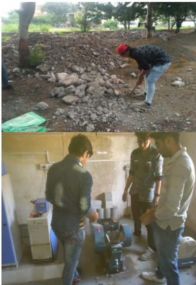
Fig. 1. Crushing wastage and demolished concrete by hammering and jaw crusher and get 20mm down aggregate
