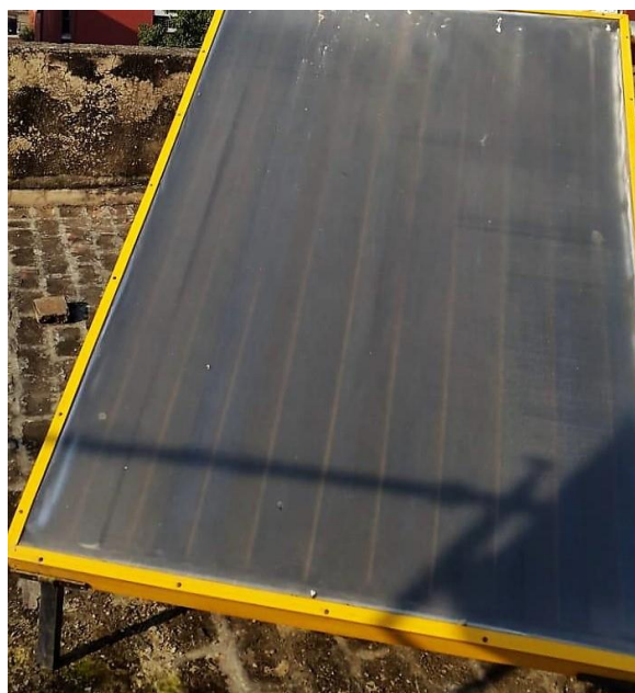
Fig. 2(a) Actual picture of flat plate collector mounted on rooftop having angle of tilt 30.76 degree.
